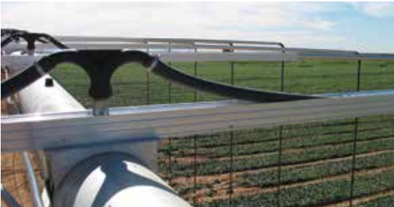
Sprinkler height can be varied by drop hose length.
